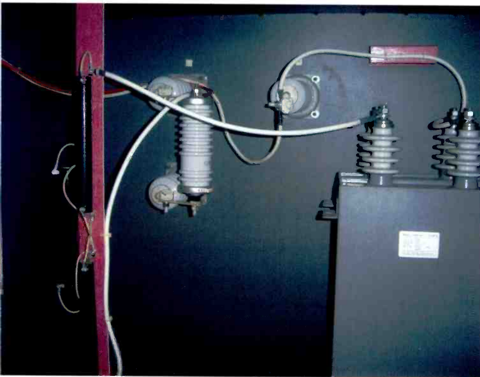
The mechanical connections inside a beam transformer should be mechanically tight in order for them to be electrically sound.
