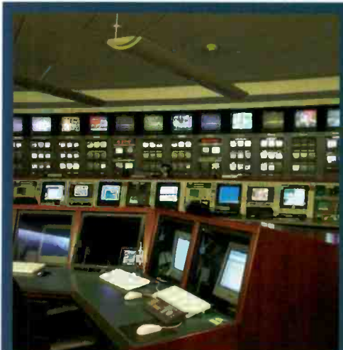
Intelsat's teleport in Ellenwood, GA, provides uplink, downlink and turnaround services to broadcast stations.
