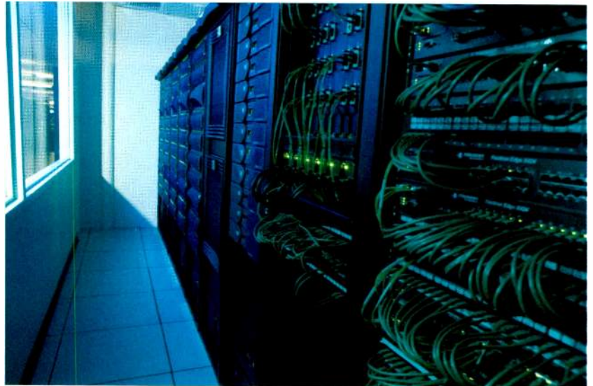
Broadcasters today often rely on internal IP-based storage and networking technology to support data rates exceeding 1.2Tb/s.
