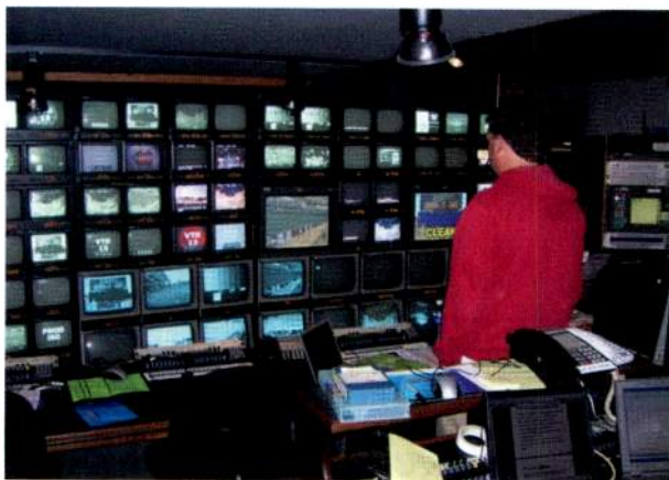
Ten Deko 3000 graphics systems were installed in mobile units and in the broadcast center at the STAPLES Center, shown here.
