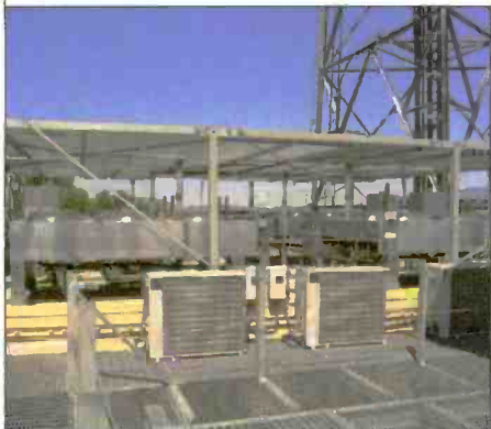
At Mount Wilson, near Los Angeles, four integrated rooftop heat exchangers provide cooling for up to eight dual-tube IOT transmitters. Photo courtesy Axcera.
