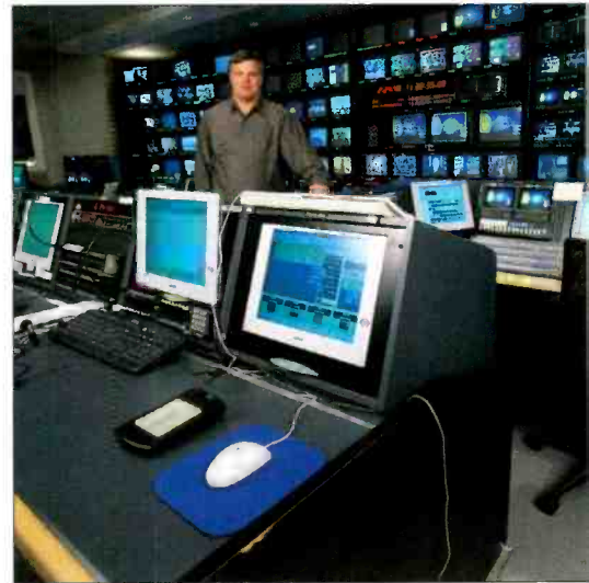
Steve Fastook, vice president of CNBC technical and commercial operations in one of three new production control rooms that include a Sony MVS-8000 switcher and Grass Valley NewsQ Pro system for preview and access to all clips within the facility.
