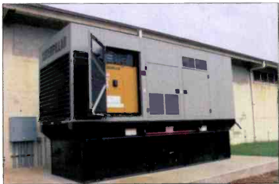
Larger generators like this outdoor stand-alone unit consume more than 80 gallons of diesel fuel an hour. This generator has a Nema 3R enclosure and base fuel tank.
