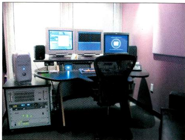
As part of an overhaul of station editing facilities, the project team installed six Avid Media Composer 1000XL nonlinear editing systems. The systems interface with an Avid Unity Media Network to allow staff members across the facility to collaborate in real time using high-bandwidth media.
