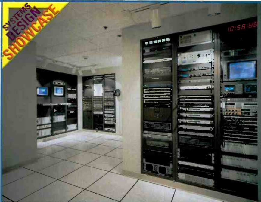
Thirty-six inch racks help support deep profile equipment. All digital audio and video signals enter the transmission area from broadcast operations through independent path routing.
