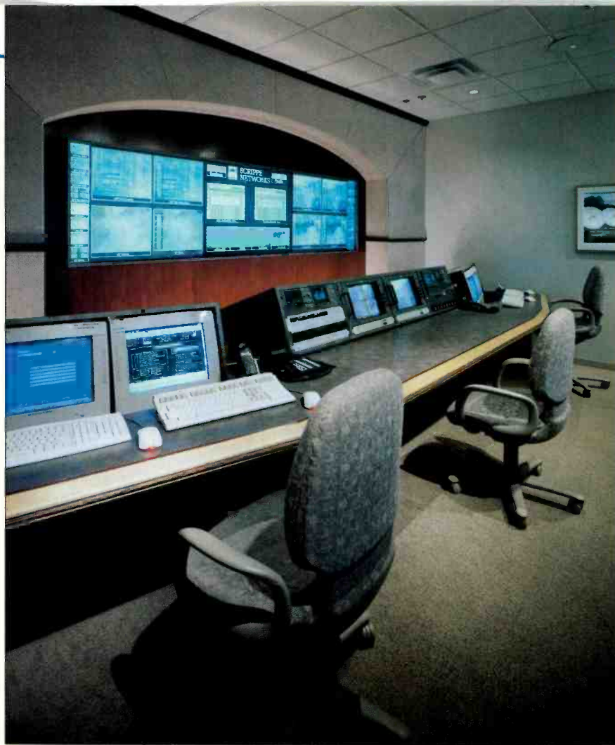
Multi-network, full transmission signal monitoring is facilitated in the transmission control room using an Avitech video command center and three Christie Digital 50-inch DLP projectors.
