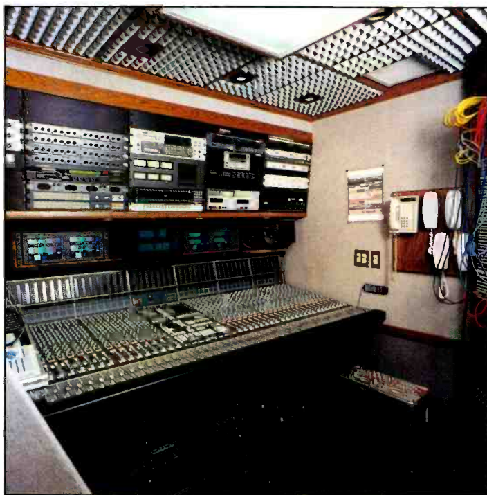
Corplex installed Solid State Logic's MTP mobile digital console in its new production truck to help customers broadcast in a range of venues.
