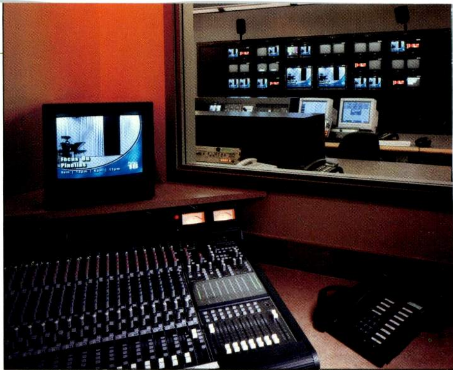
Although both channels reside in the same facility and use identical equipment, they have separate control rooms, studios and offices. In addition, a tight budget forced the county to choose cost-effective equipment.
