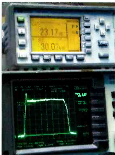
Figure 1. Spectrum analyzer and power meter showing the results of 8VSB modulation through a TH770/TH18770 system at 30kW (avg.) output power.
