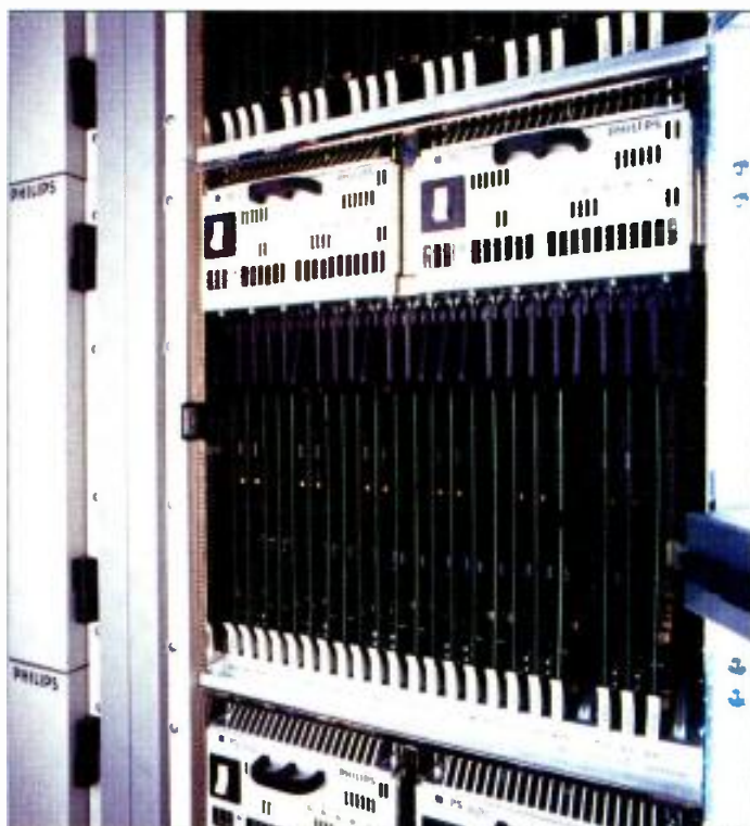
Large routing systems can take considerable rack space. Be sure to plan for sufficient rack space and cooling for the system chosen.
