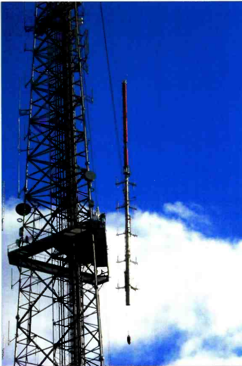
WRC, Washington, DC, chose to stack its NTSC antenna at 587 feet and its digital antenna at 637 feet. Shown are the antennas being raised into position.
