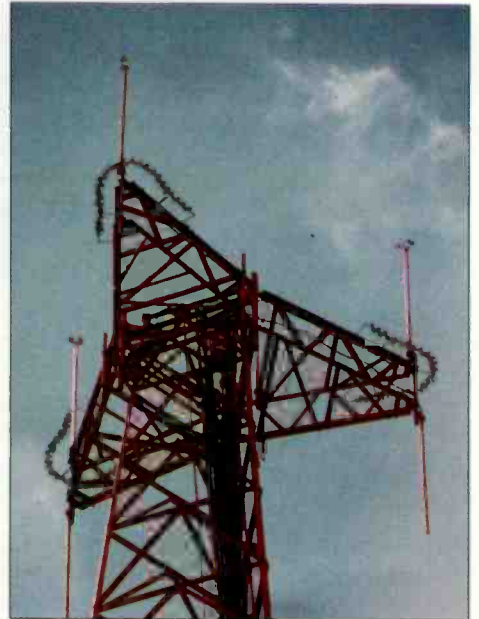
This cellular tower is equipped with lightning-protection products placed at areas of maximum curvature — on each vertex of the cantilebra structure and atop each antenna stake. (Courtesy of Lightning Master Corporation.)
