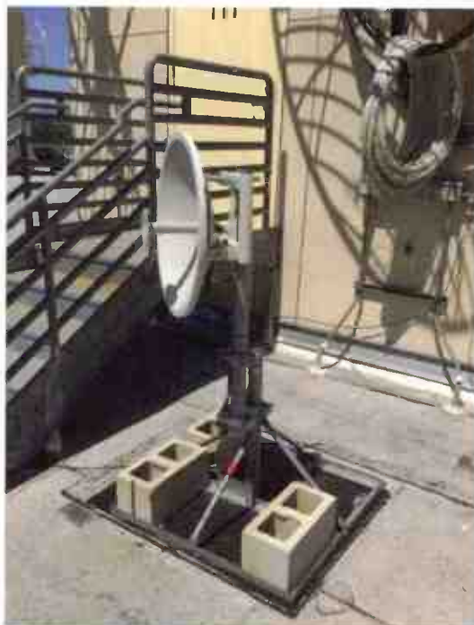
One advantage of the current crop of ISM radio systems is their diminutive size, which can be accommodated by a simple non-penetrating roof mount, as shown.
