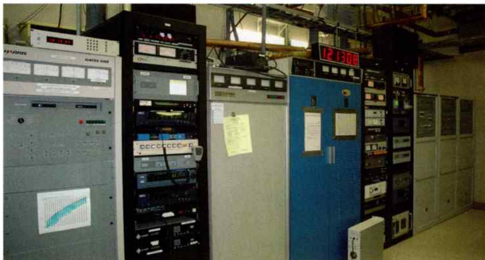
Old transmitters, like the Gates or Harris ones shown in the middle above, can serve for years when some TLC is applied.
