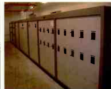
CUSTOM PHASOR INSTALLATION
