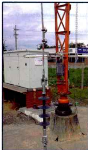
MODEL KSA-VCTB-10 KINSTAR LOW PROFILE ANTENNA ON THE AIR IN COLOMBIA, SOUTH AMERICA
