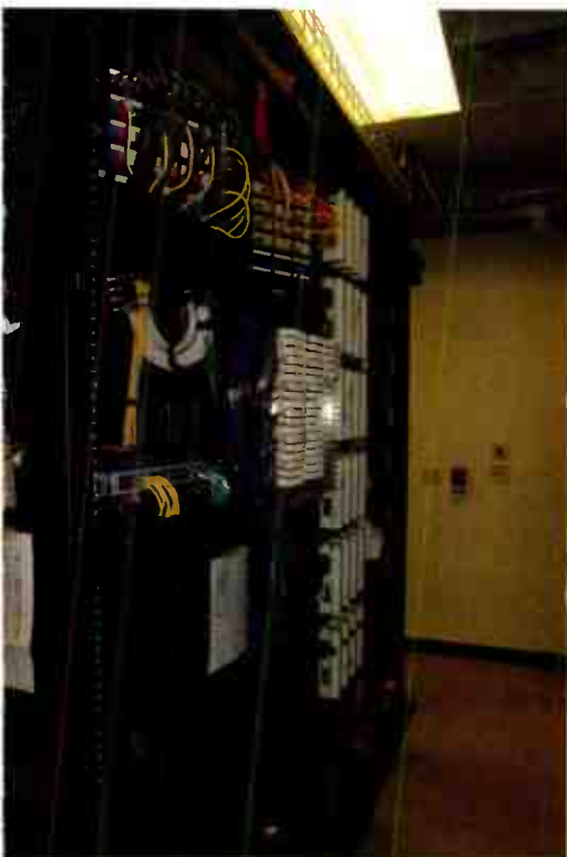
Wire management racks were used for Ethernet and digital audio cross connects.
