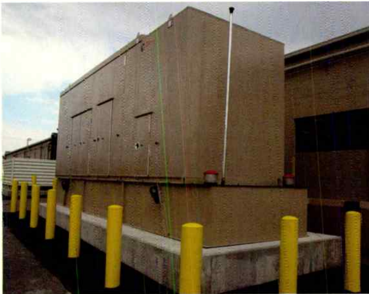
An Onan 750kW generator was installed to provide auxiliary power to Dial Global's network operations center.
