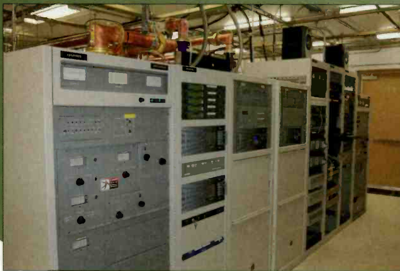
The new transmitter line-up
