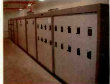
CUSTOM PHASOR INSTALLATION
