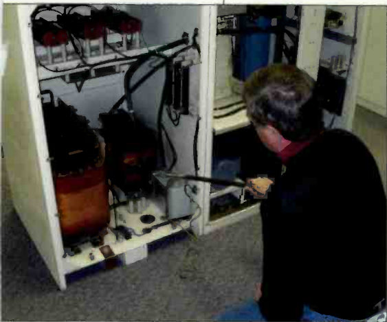
Always verify that no voltage is present before going in.
