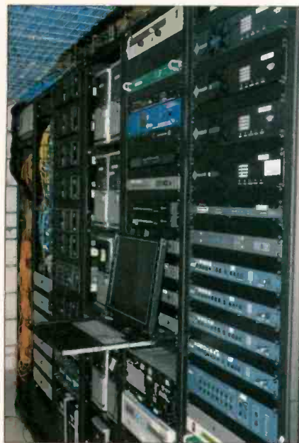
The 8' racks in the TOC
