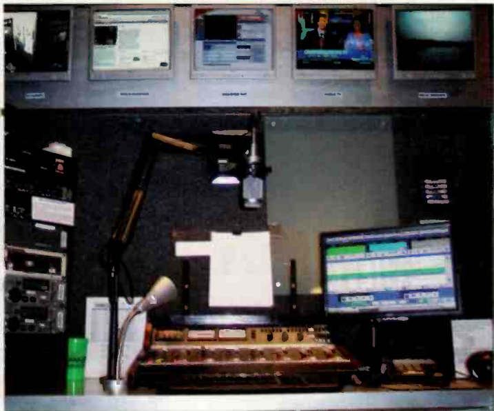
The new operator's position after the remodeling.
