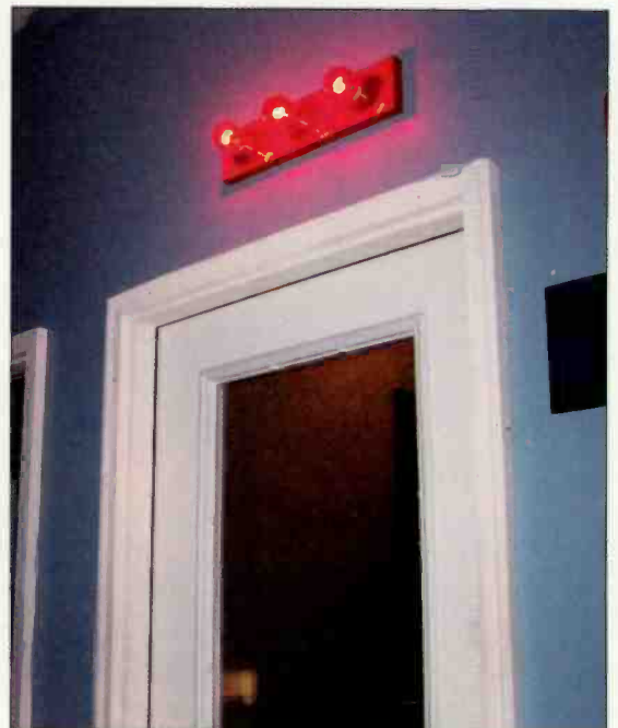
The existing door was re-used. A vanity light was adapted to serve as an on-air light.
