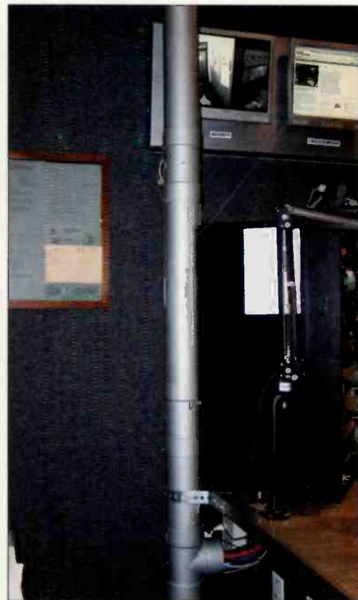
Painted silver, PVC pipe was used to route cable from the ceiling to the furniture.
