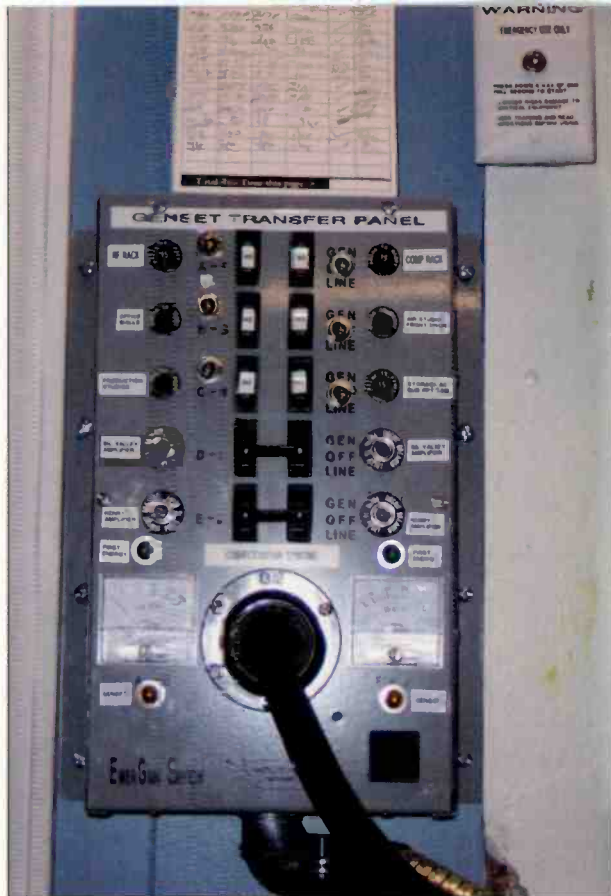
The custom generator panel provides flexible control of ac power.
