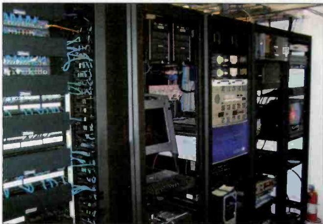
A look at master control with Cat-5 connects, SAS router, OMT logger, GPS lock and NAS drives for network audio storage.
