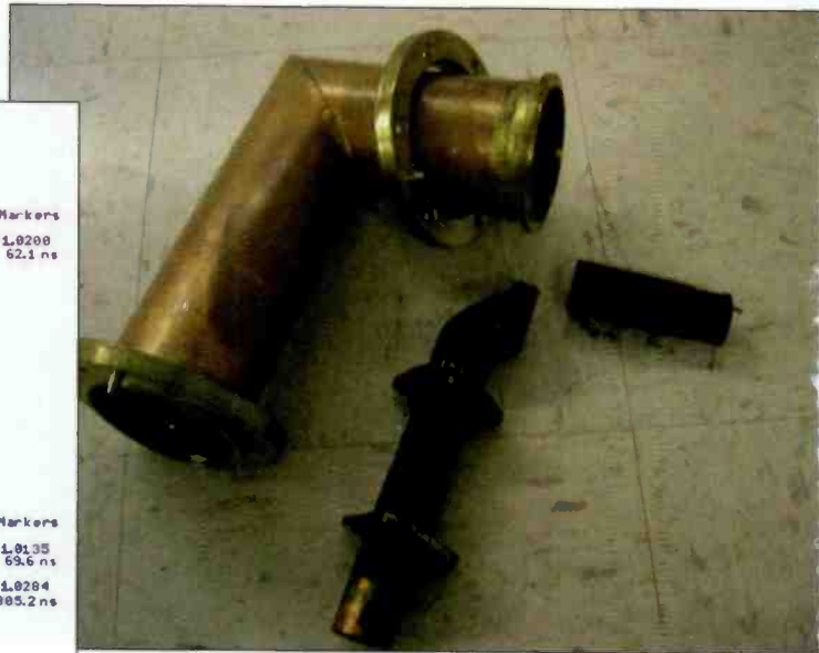
Figure 5. Opening this elbow revealed an obvious problem.
