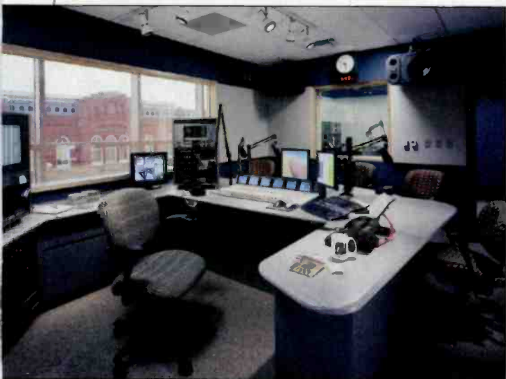
The main air studio is built around Wheatstone G5/20 control surfaces. Photo by Tom Crane Photography, courtesy of Burt Hill Kosar Rittelmann Associates.
