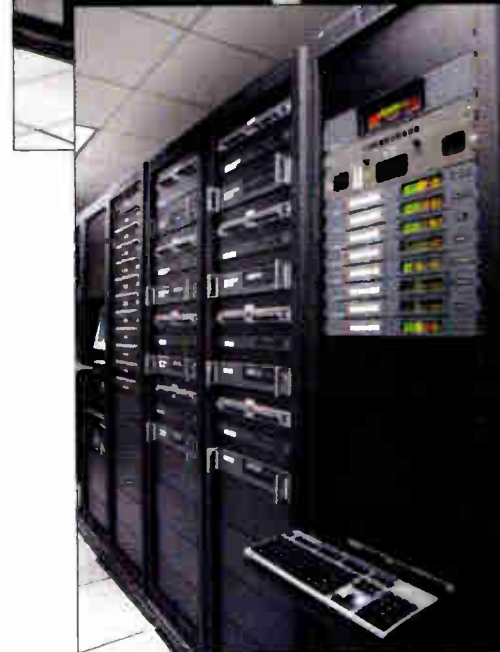
The master control room houses rows of racks. Much of the wiring was completed off-site and then installed later.
