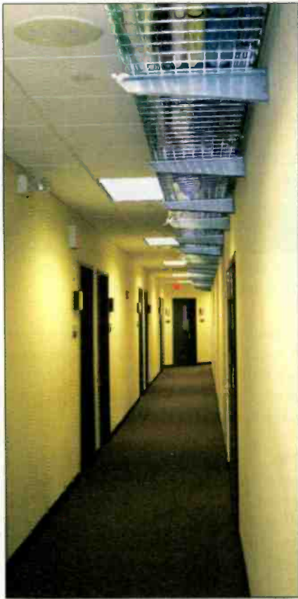
The cable trough runs down the hall, so neat cable installation was important.
