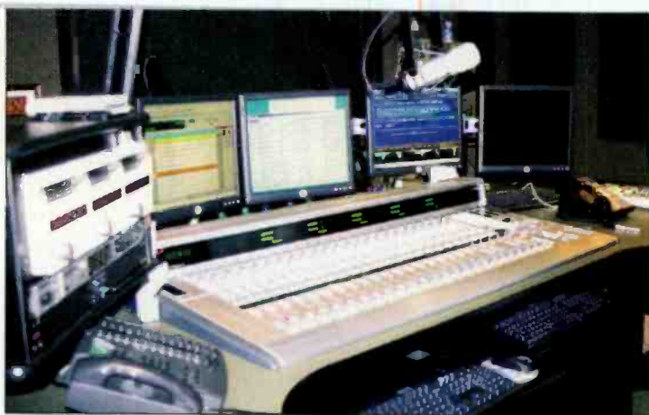
All the control rooms have layouts similar to the WEBN control room shown here.
