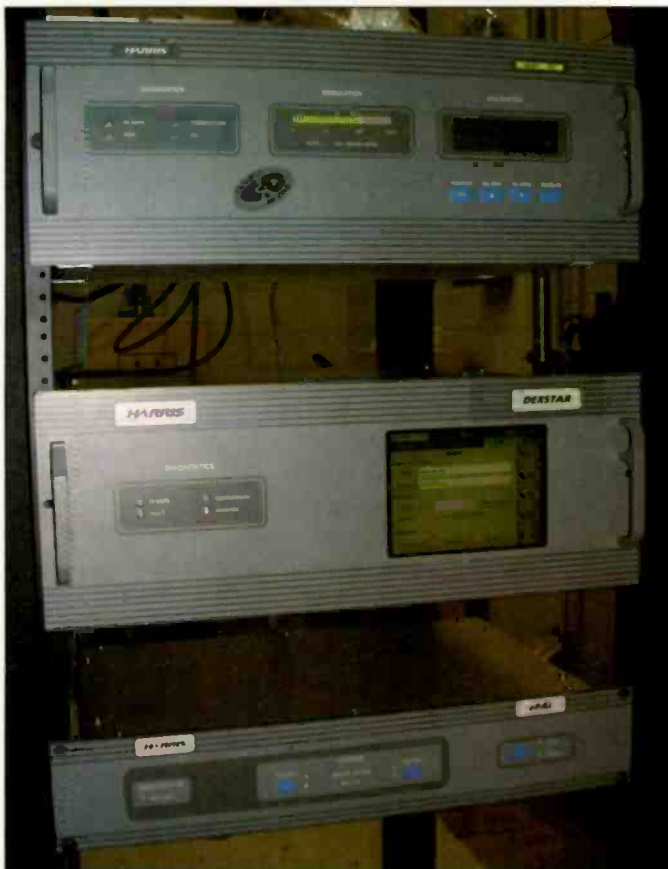
The exciter rack with a Harris Digit exciter, Dexstar IBOC exciter and Epal audio interface.
