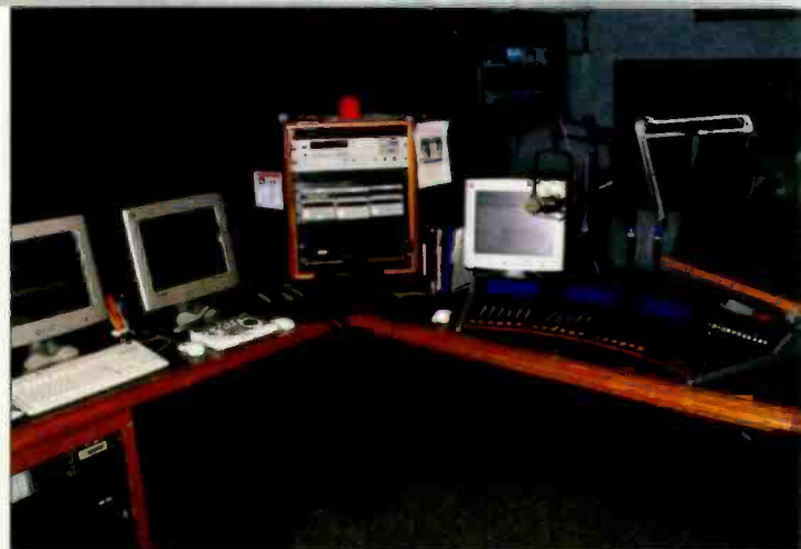
Each studio has a conventional layout, but the integration of routing and control adds to the flexibility.
