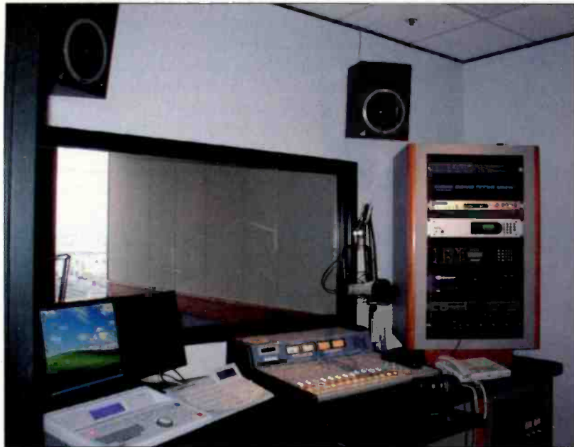
The control room oversees the talk studio, and was designed to maximize its flexibility in a limited area.
