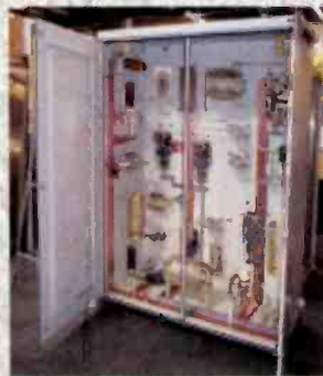
DIRECTIONAL ARRAY ANTENNA TUNING UNIT GAITHERSBURG, MD
