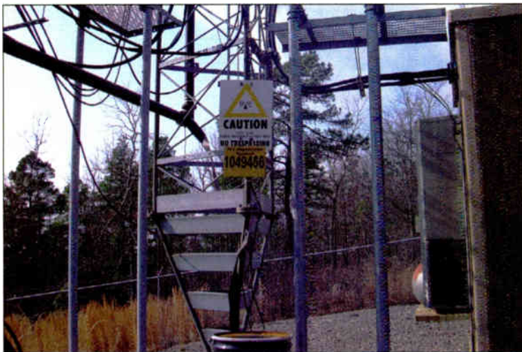
As specified by the FCC, proper signs should be posted on the tower or near it, aside from those in plain view by the public at the gate of the premises.
