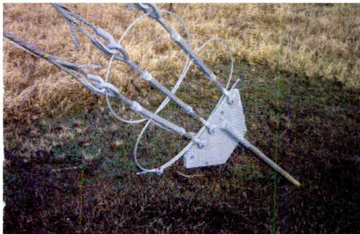
Guy anchor showing the turnbuckle safety in figure-eight formation as required by TIA/EIA 222.
