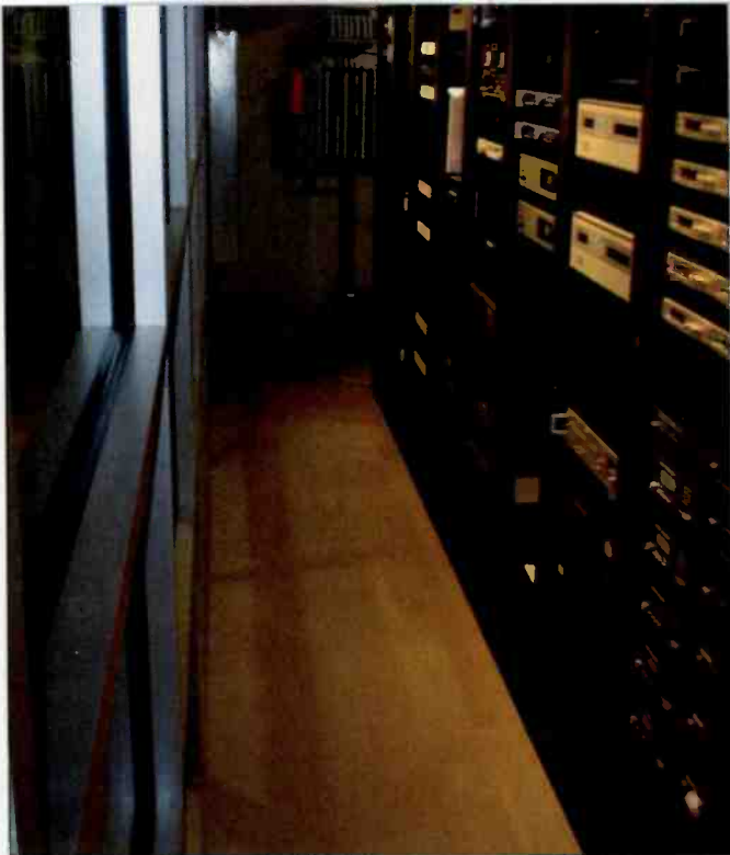
The rack room is behind a glass wall facing into the hallway.
