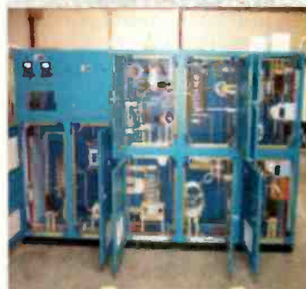
THREE TOWER AM 50kW NDA-D / DA-N DIRECTIONAL ANTENNA SYSTEM ST PAUL, MN.
