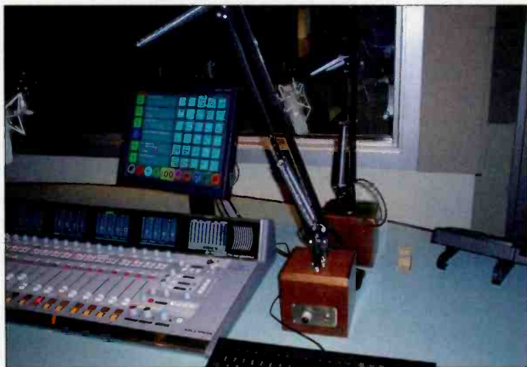
Another view of the Super Talk 99.7 WTN control room.
