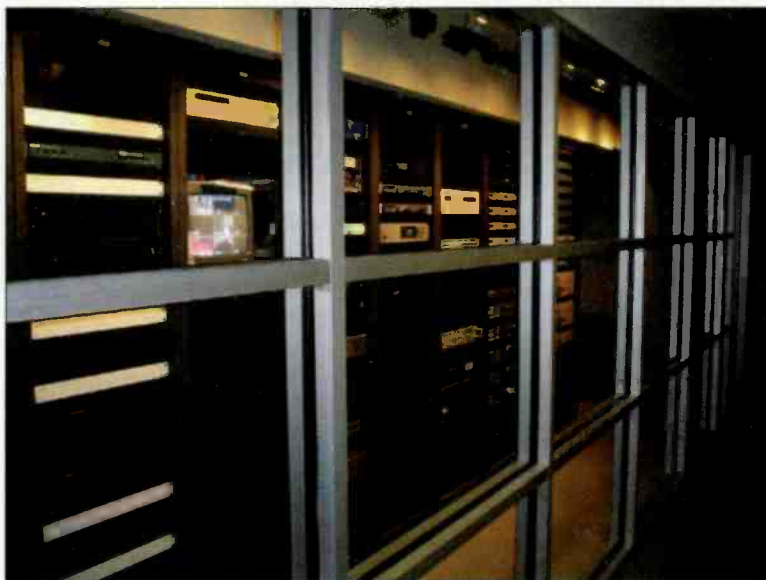
Most Cumulus facility installations now place the rack room behind a glass wall to provide an easy view of the equipment, which is impressive to non-technical visitors.
