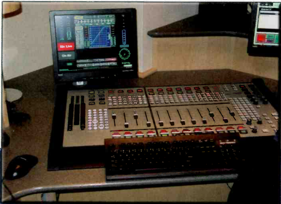
The console in the WCSX production studio. The monitor shows the DSP audio compressor/expander.
