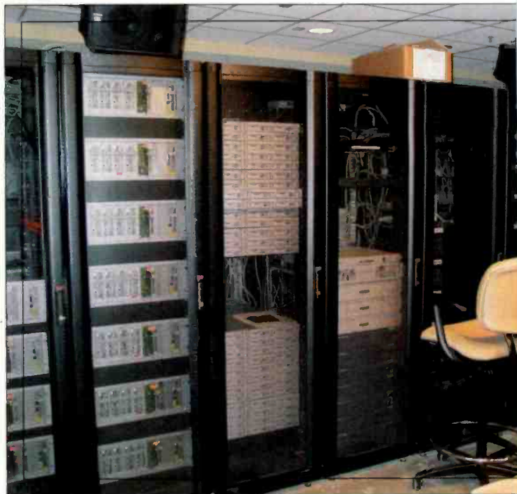
Looking into the technical operations center showing the Raritan KVM cross-point switcher, Klotz Vadis frames and Gateway servers.
