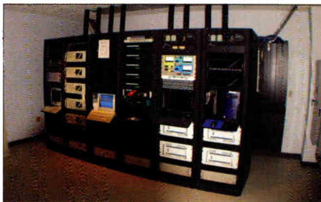
The centralized equipment room houses the Wheatstone Bridge 2001. The studios are wired with a Wiremax Studio Interface System.
