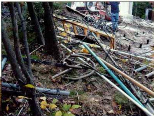
A fallen tower is one of the most severe emergencies.
