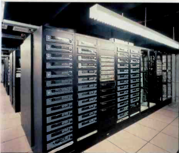
The rack room houses all the audio processing, audio servers and encoding equipment for the entire facility.
