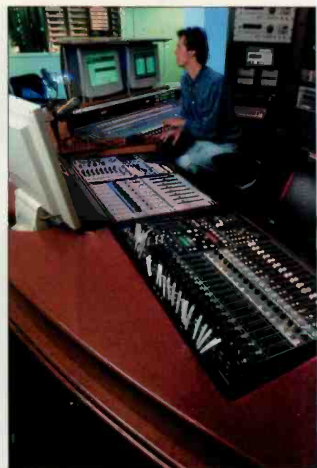
Some studios have two consoles for on-air or production applications.
