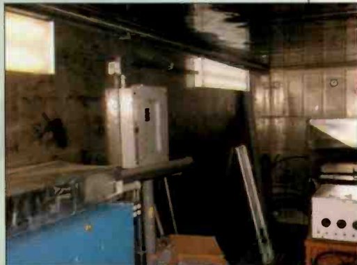
Inside the generator container.
