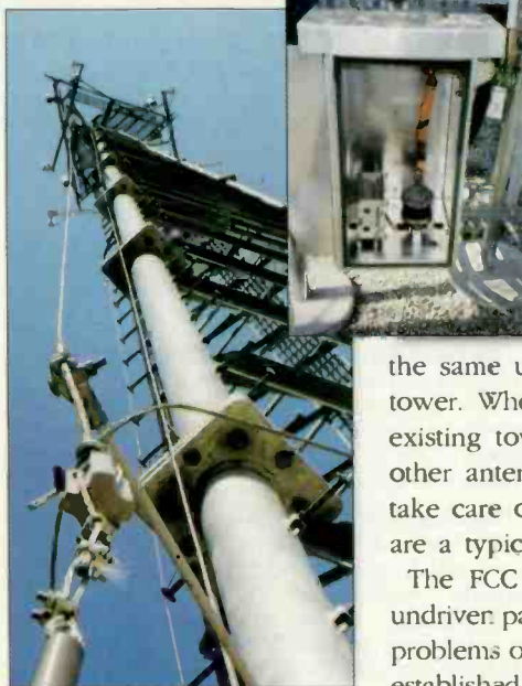
Structures built within an AM station's coverage may require detuning so they appear invisible to the AM station.
