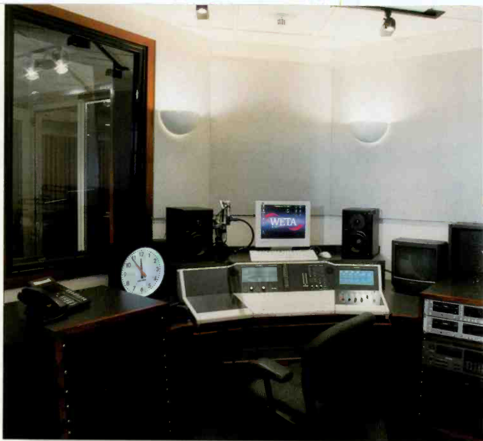
The edit rooms are smaller than the other studios but just as functional. Each of WETA-FM's three edit rooms is built around a Studer audio console.
