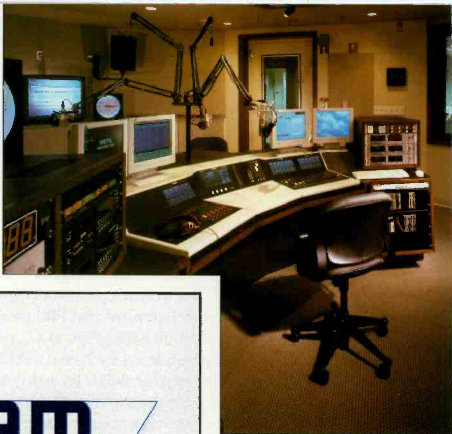
The heart of the station, the WETA-FM on-air studio is ergonomically designed to ensure employee comfort.
