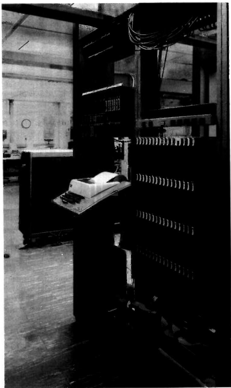
Fig. 3—Microprocessor Controlled Load Box.
