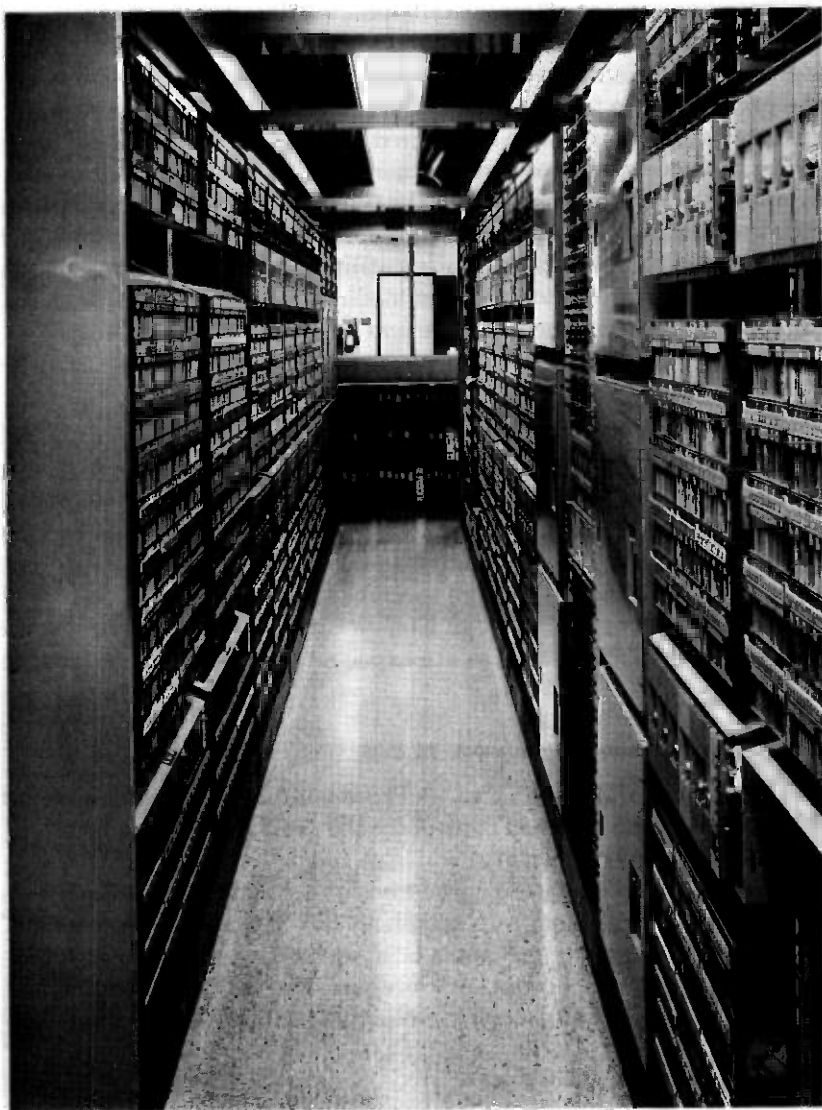
Fig. 3—1A processor in No. 4 ESS (Chicago toll office).
