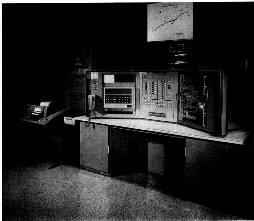
Fig. 4—Transmission surveillance center at Xenia, Ohio, station.
