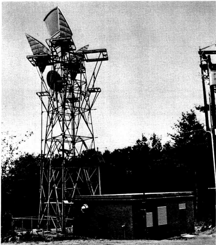
Fig. 4—Dunbarton, New Hampshire, combined TH-3 and TJ radio repeater station.
