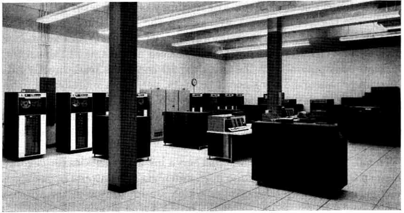
Fig. 2 — Two computing systems with four tape units each; three cabinets between tape units contain tape switching equipment.
