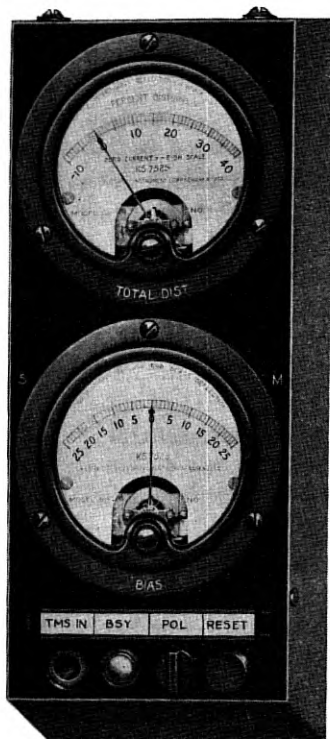
Fig. 3—Meters and control apparatus at telegraph board.
