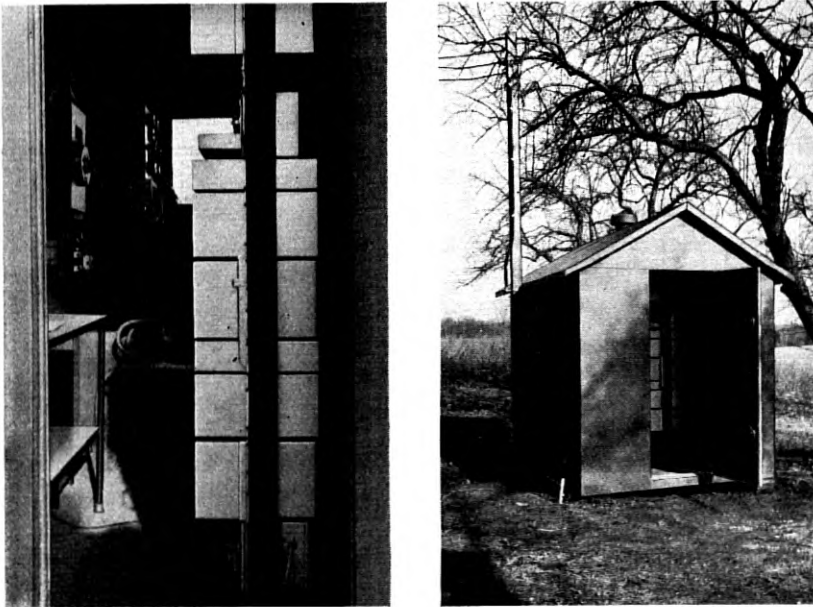
Fig. 9—Interior and exterior of special intermediate repeater station at Abingdon, Md.
