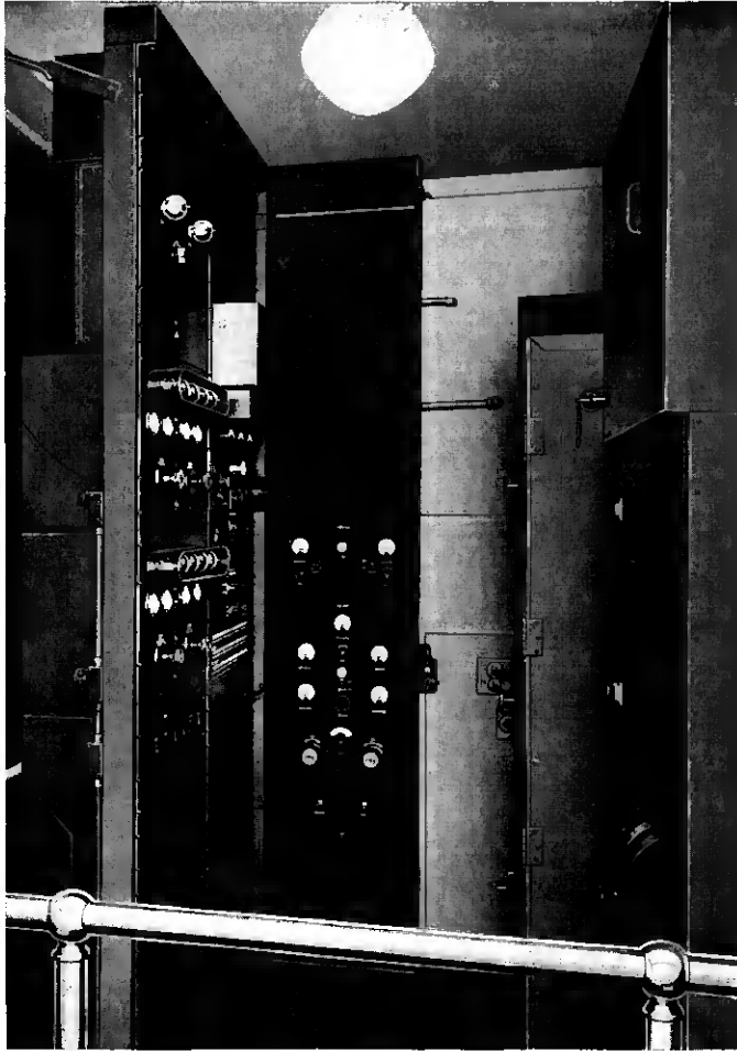
Fig. 11—Control apparatus panels associated with one terminal of the television apparatus.
