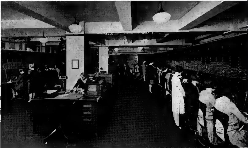
Fig. 8.—Private branch exchange—1600 stations, 148 lines to Central Office, 151 tie trunks to other private branch exchanges, 42 switchboard positions, 60 operators and 24 hour service.
