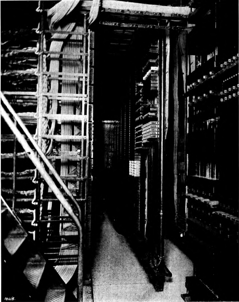
Fig. 1—Relays in a local manual office
