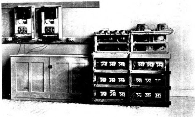
Fig. 1—Box Type Repeater Installation
