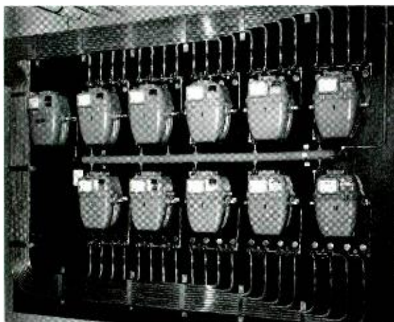
Former arrangement for monitoring gas pressure in cables. In addition to requiring daily readings of each counter, these meters occupy considerably more space than do the new design meter panels.
