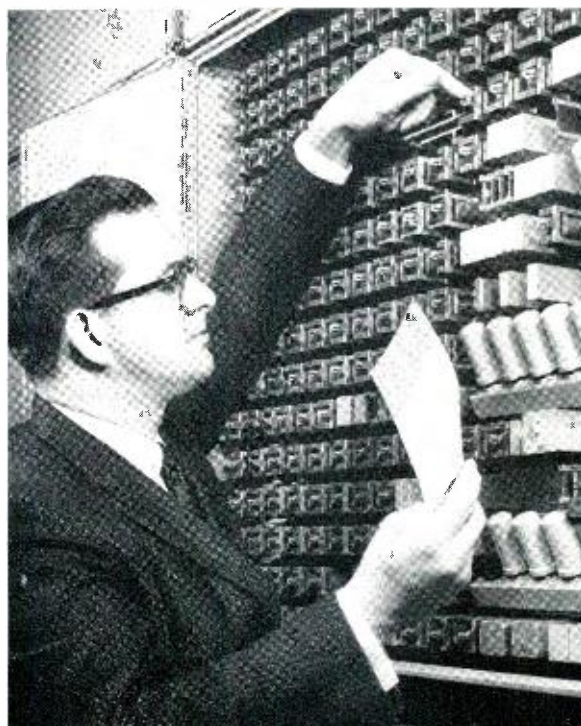
T. P. McGuinness checks a relay that failed in the sender circuit during a service call. Trouble-recorder card records progress of call and indicates trouble items detected by self-checking features.
