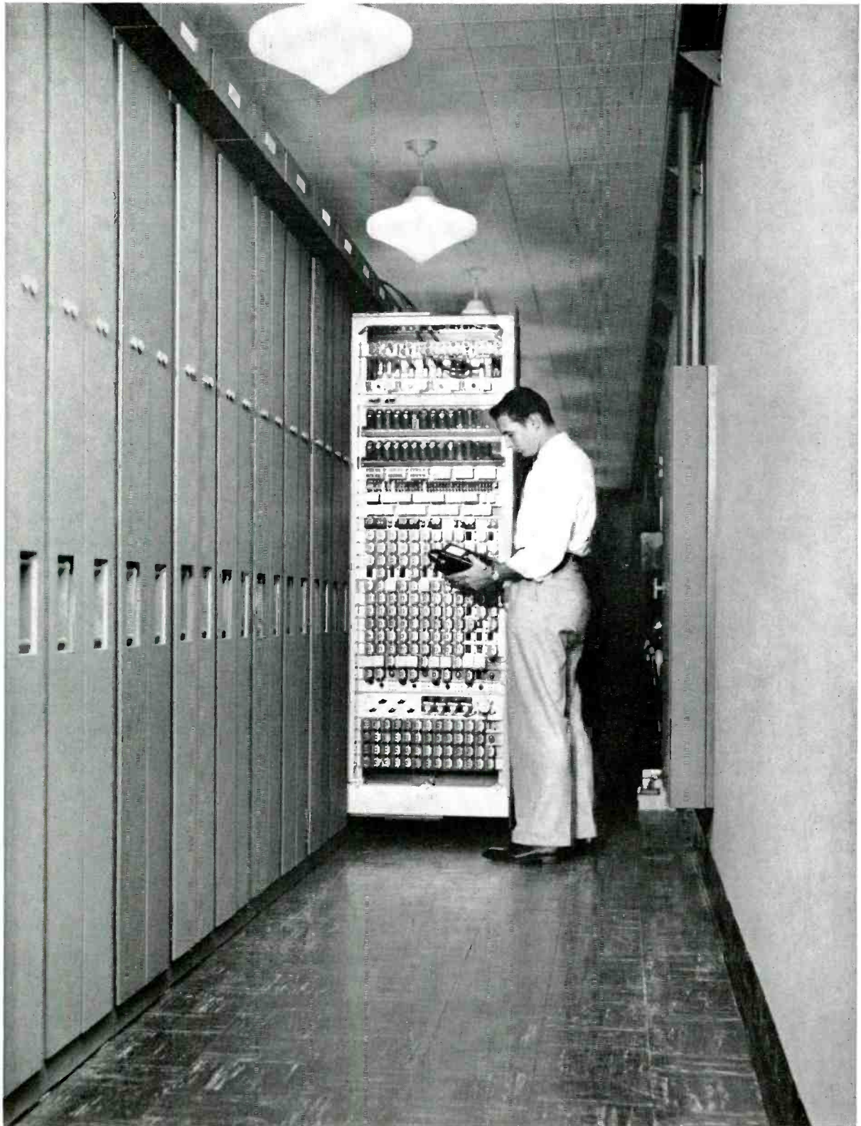
J. W. Emmons, of the New Jersey Bell Telephone Company checks voltages on equipment in lineup of "outgoing" cabinets. Equipment can be easily added or removed according to needs of the office.
