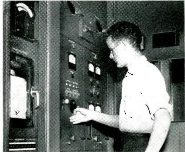
H. B. Burton, Eastern Telephone & Telegraph Co. tester, adjusting the autotransformer handwheel in a regulator bay at Clarendville. Part of the associated common-control bay can be seen at left.
