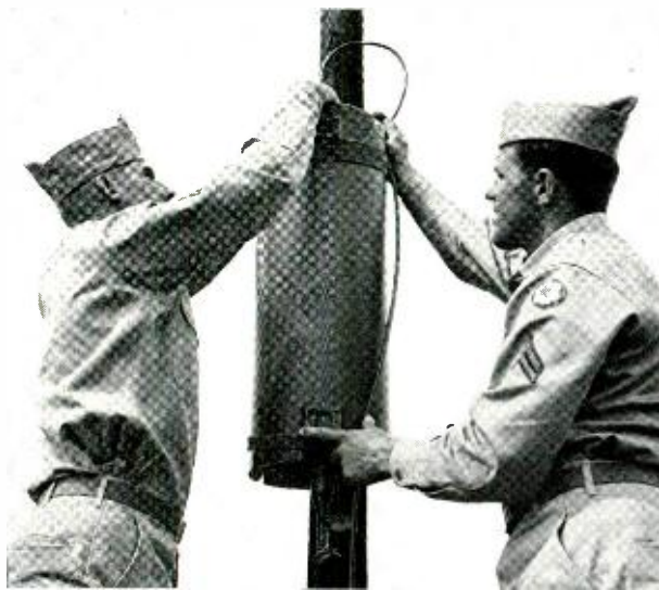
Fig. 1 — Mounting AN/TCC-11 unattended repeater on a pole. This repeater unit can also be placed on the ground along the cable run.
