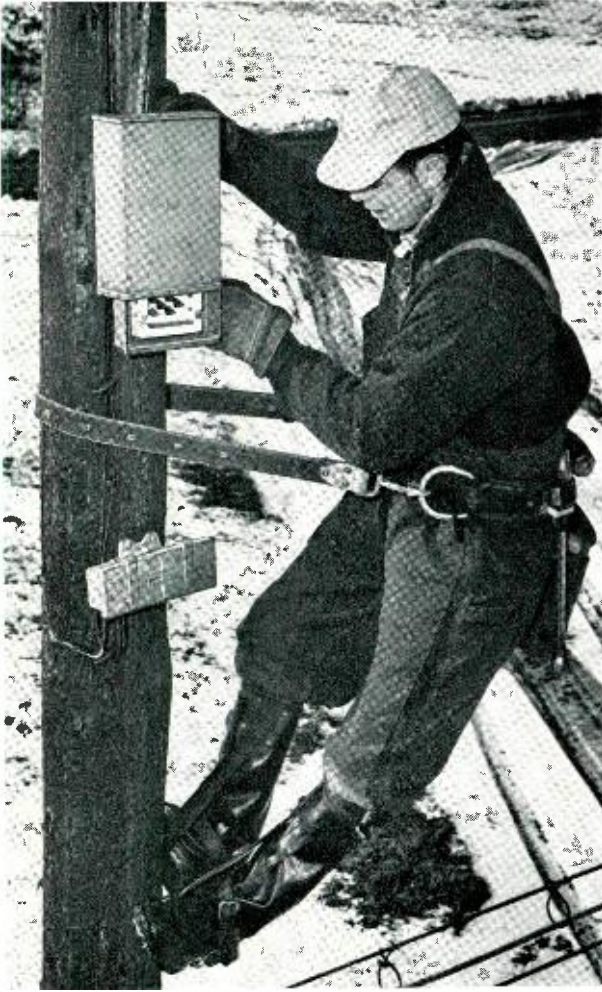
Fig. 5 — Older F-type cable terminal cover raised by John Apgar to show faceplate and binding posts. Protectors are housed in mounting underneath.
