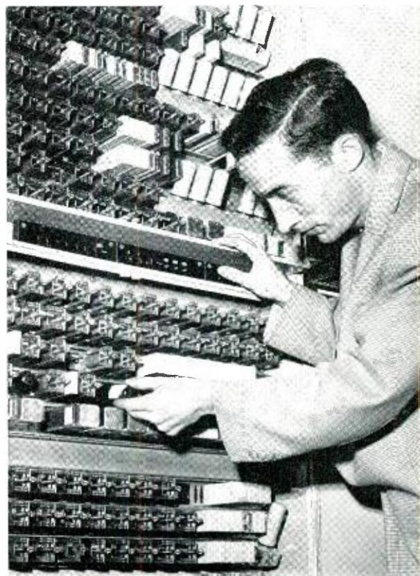
Fig. 2 — M. J. Norton replaces a gas-tube in a laboratory model of a 4A decoder.
