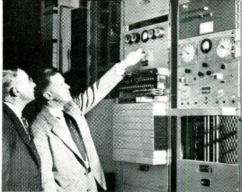
Fig. 4—Vincent Amoroso of the New York Telephone Company and A. E. Gerbore of the Laboratories inspect the time-of-day equipment in New York City.
