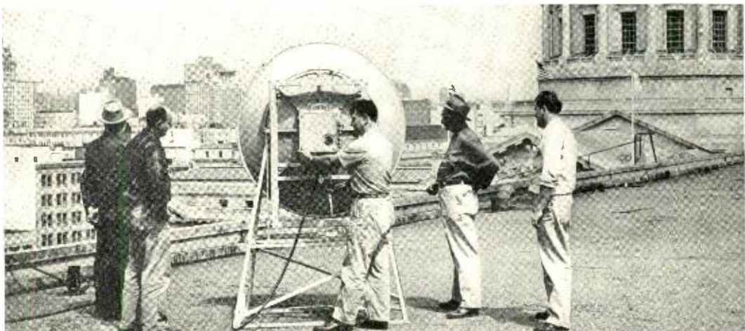
Pacific Company engineers install the antenna which was used to beam television signals from the roof of the Opera House into the transcontinental radio relay system.
